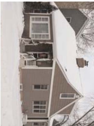
4161 Toledo Avenue South Jill and Michael Riley kitchen, family room and mudroom addition
